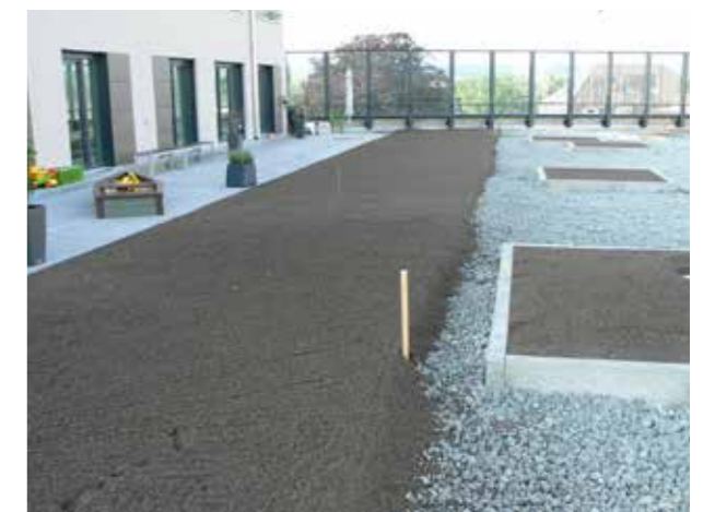
EDEKA Verbraucherzentrum in Konstanz, layout of paths and green areas with a total of 2'000 m 3 MISAPOR
